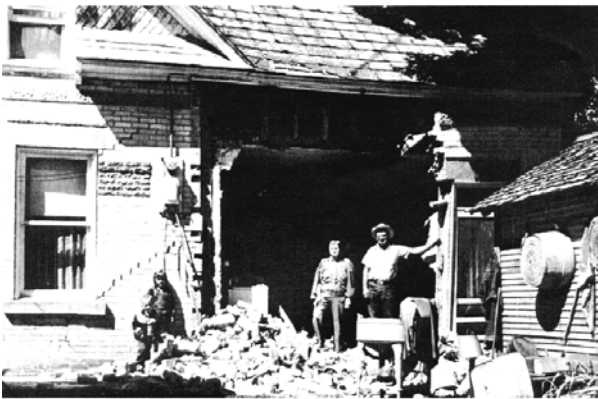
Damage to an unreinforced brick house in the 1962 Richmond earthquake
